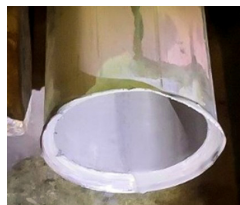
Figure 3: View of the cut on the 7-inch CRA-110 liner
